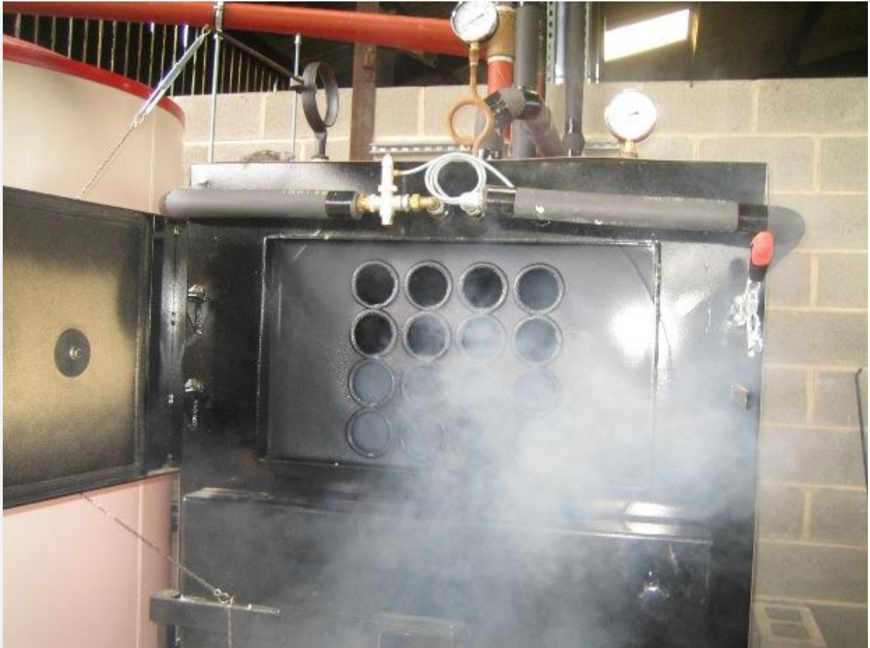
The bio mass boiler at Beechenhill B&B
